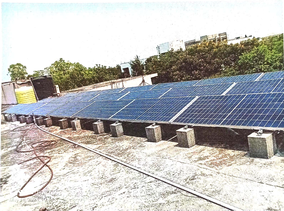
Figure 14 Solar PV System
